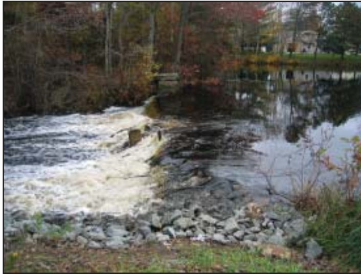
The firm handled dam inspection, permitting and hydrology analysis for the Old Forge Lake Dam.
